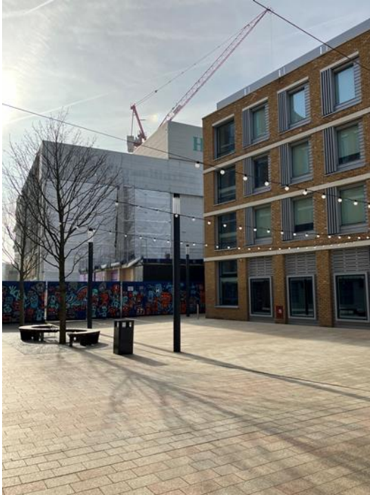
Image (left): View of partially constructed Block C podium with former Printworks building in the background.
